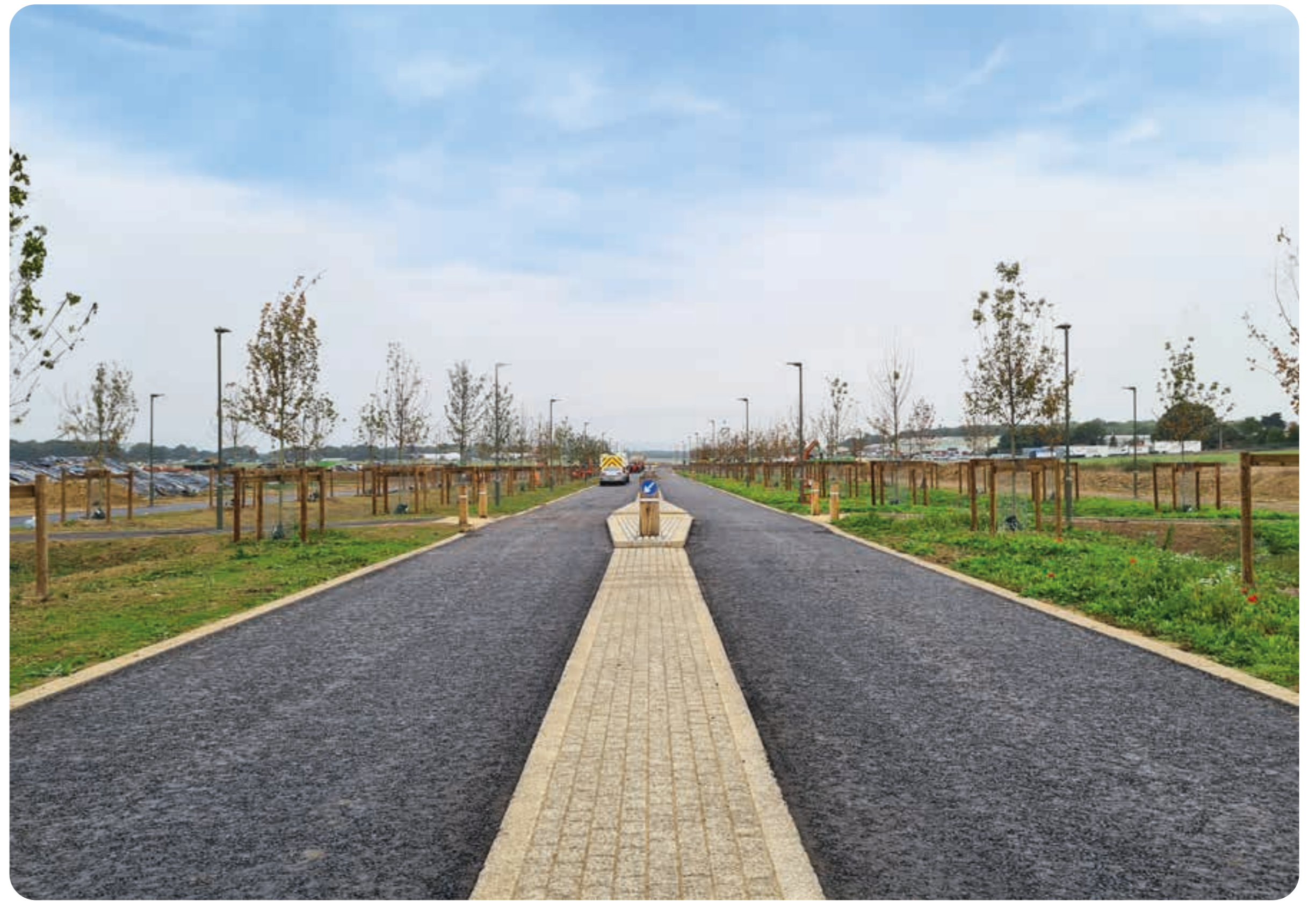
Photo showing newly completed main access road from the A281 - Canada Avenue
